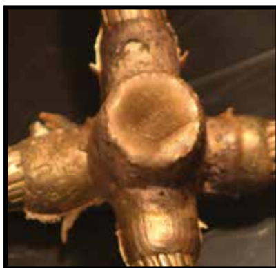
Image 3: A worn or incorrect mold was used, allowing leakage around conductor. The fill in this connection is sufficient to make it as acceptable.
