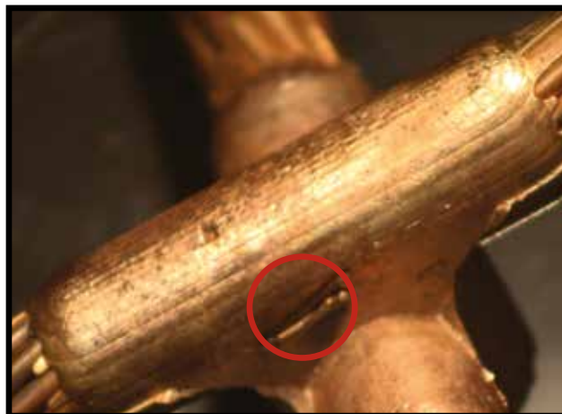
Image 7: Poor connectivity. Visible wire shown in weld.
